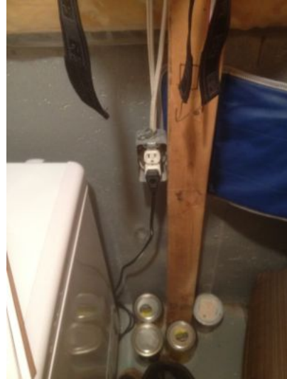
SAFETY CONCERN: Missing cover plates at multiple outlets and light switches. Repair as needed.
