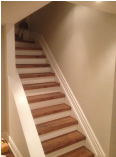
Recommend hand rails leading to basement.
