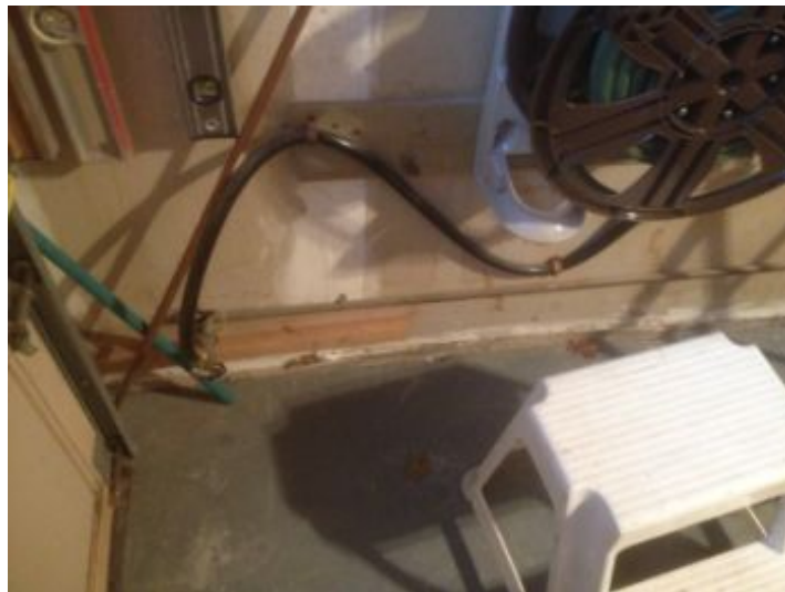
Insulation advised for pipes at unheated areas.
