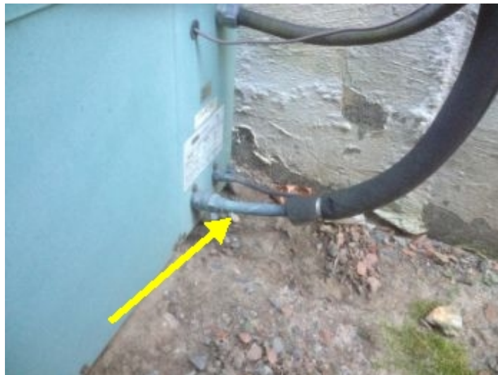
The insulation is missing or damaged at exterior refrigerant line.
