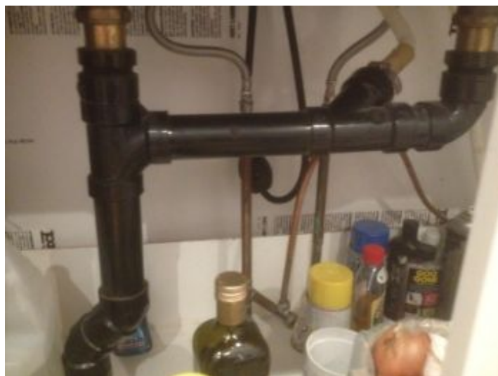
No drain trap observed in hall bath
