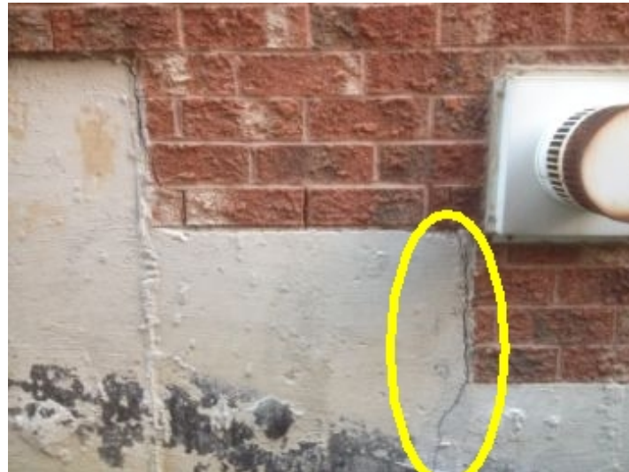
Some minor cracks from settling noted
