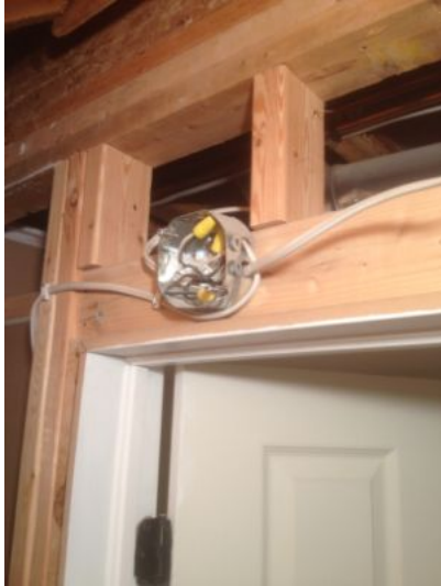
SAFETY CONCERN: Missing cover plates at multiple outlets and light switches. Repair as needed.
